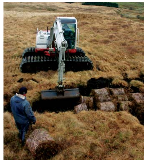
BLOCKING DRAINAGE 'GRIPS'
