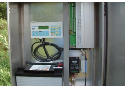
Flow metre station, close view of the cabinet
