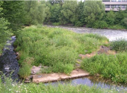
Fish by-pass close to municipality of Alfeld (source: Micheal Jürging, agwa)
