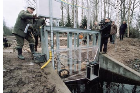
At the Finsjö fishbypass an advanced fish counter and infrared scanner was installed.
