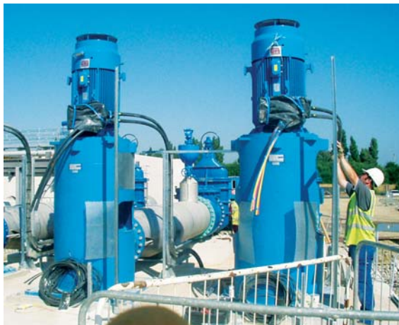
MWH AND UU ARE MANAGING A MASSIVE PROGRAMME OF INVESTMENT IN THE NORTHWEST WATER INFRASTRUCTURE
