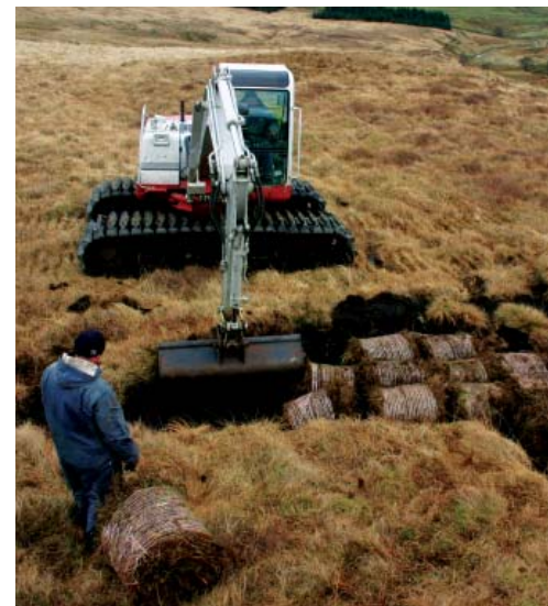
BLOCKING DRAINAGE 'GRIPS'
